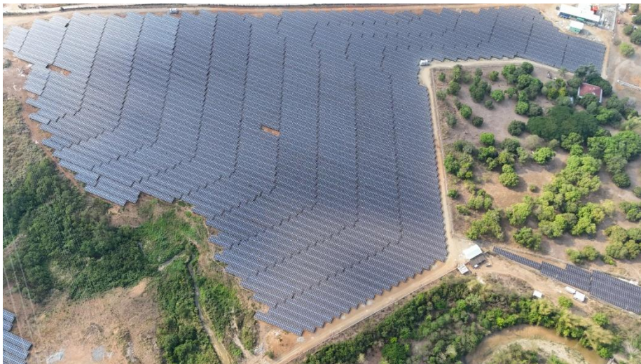
Physically completed in the fourth quarter of 2025, the BSPP utilizes 35,350 photovoltaic modules from Trina Solar, 58 Sungrow inverters, and can generate 41,000 MWh of power annually while reducing carbon emissions by 29,056 metric tons.
