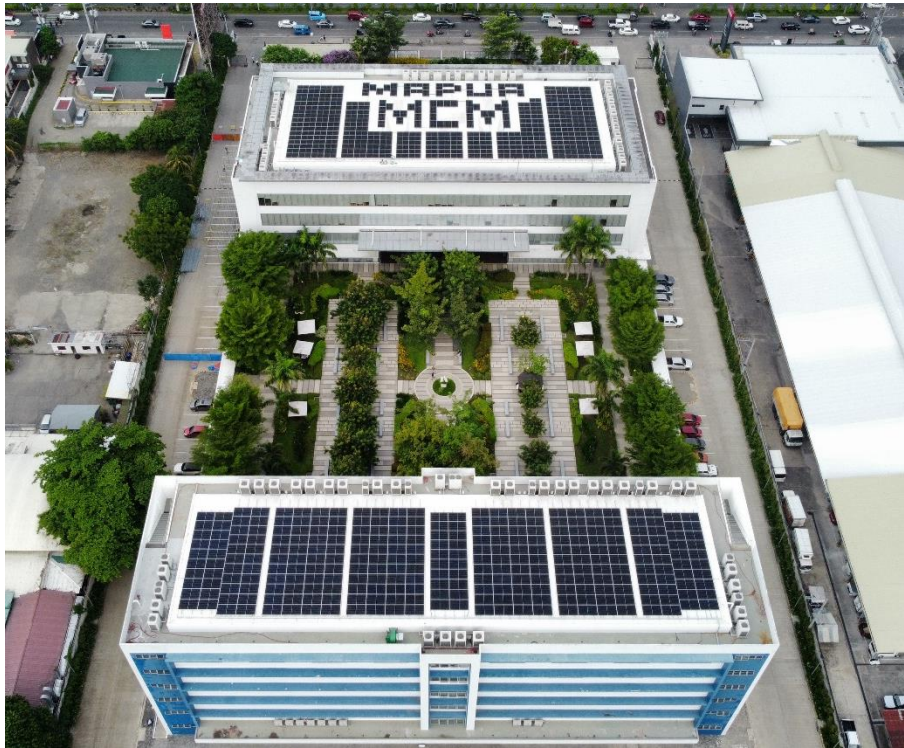
360KWp MMCM Solar Power Project powers up the school's facilities with clean and renewable energy
